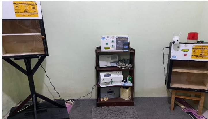
Figure 6. Emergency Tower System
