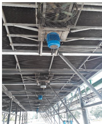
Gambar 1. Kondisi motor ACWC (Air Cooled Water Cooler ) di PLTGU IP Grati blok 1
